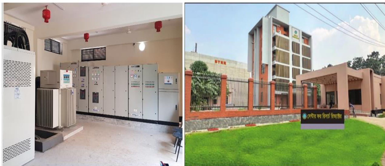
Fig. 3: 1250 kVA Electrical Sub-station (3a, left), and Outside View of CRR (3b).
