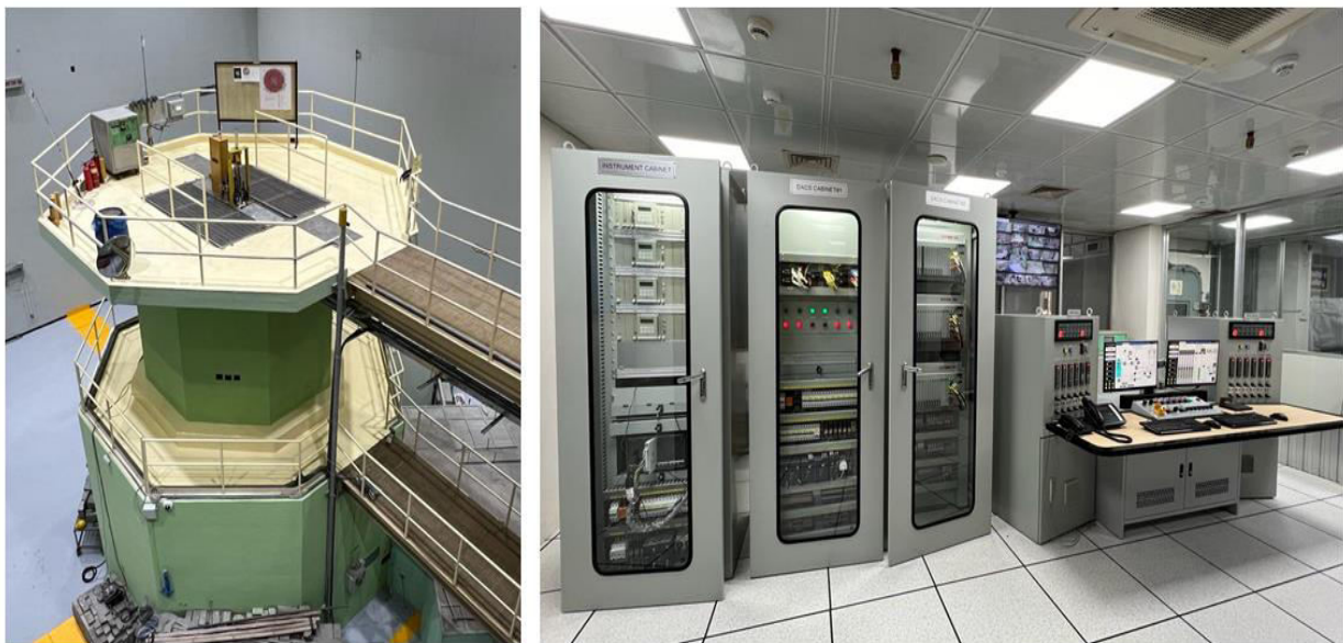
Fig. 1: Reactor Shield Structure (1a, left) and Reactor Digital I & C System (1b, right).
