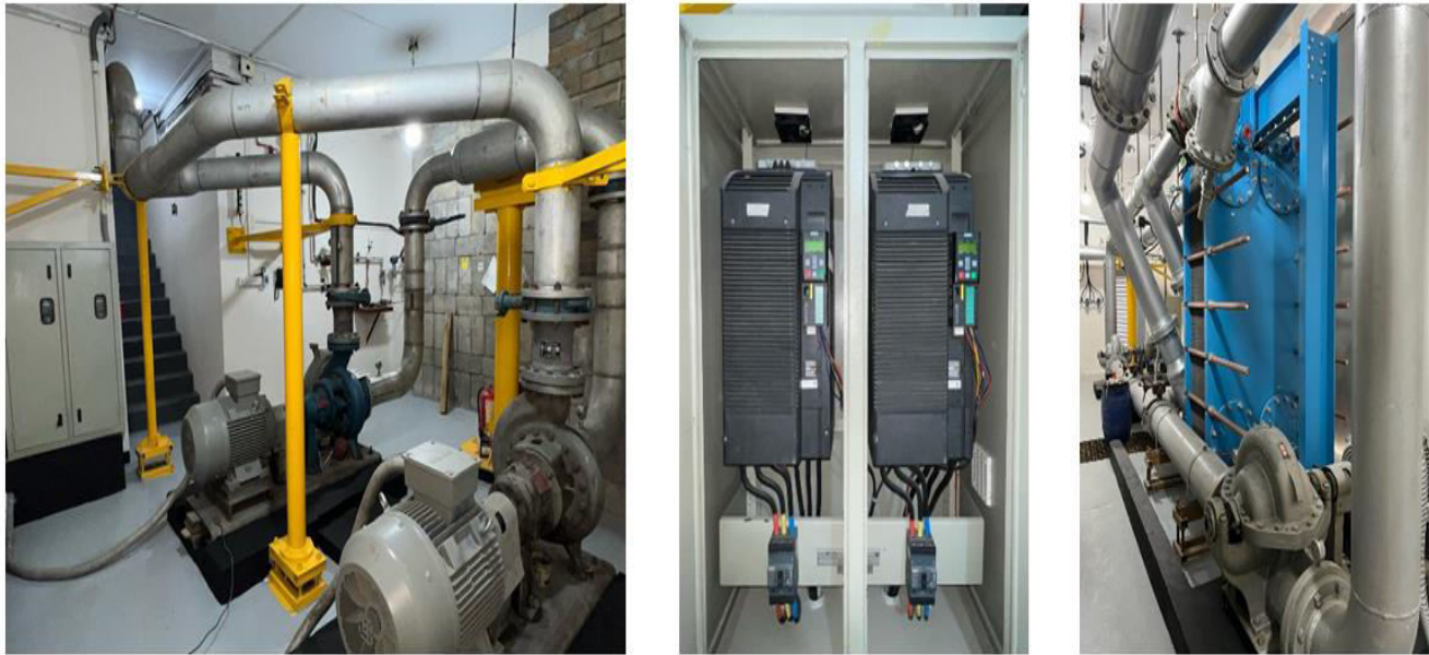
Fig. 2: Primary Cooling System Pumps (2a, left), VFD (2b, middle), and Heat Exchanger (2c, right).
